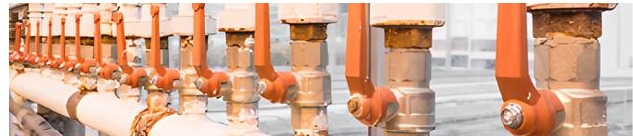
► Scaling and Corrosion Analysis of Piping Equipment
